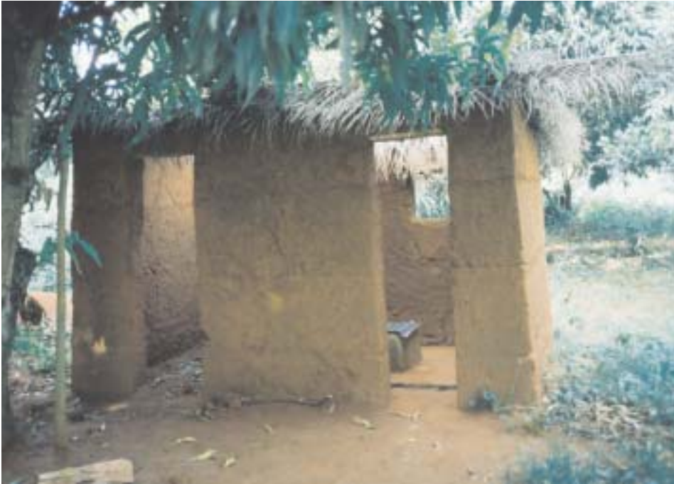
A new latrine under construction, using local materials, and adopted to incorporate a bath cabin.
